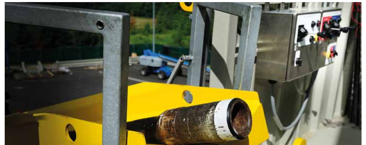
Wired control panel at V-Door
