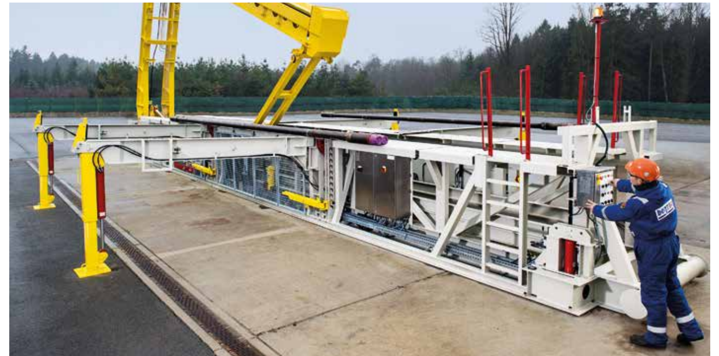
Local control panel
